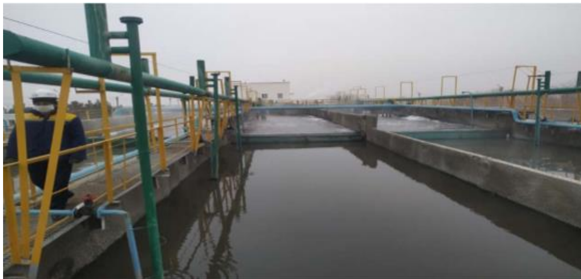
Figure 1. Aerotents that undergo primary purification from petroleum products
