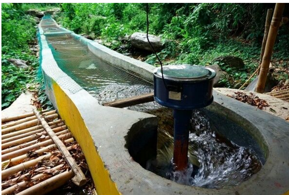
Picture 1 micro hydroelectric power station
